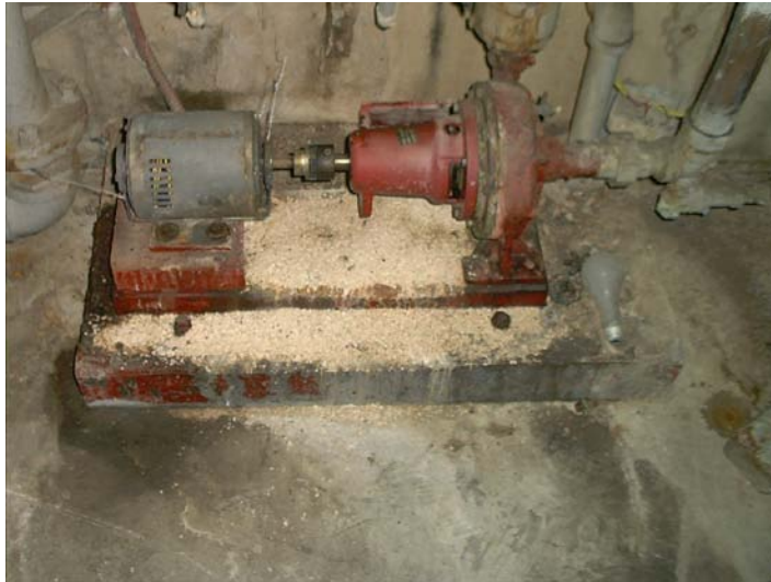
Fig. 1-4: Leaky Pumps and Valves
