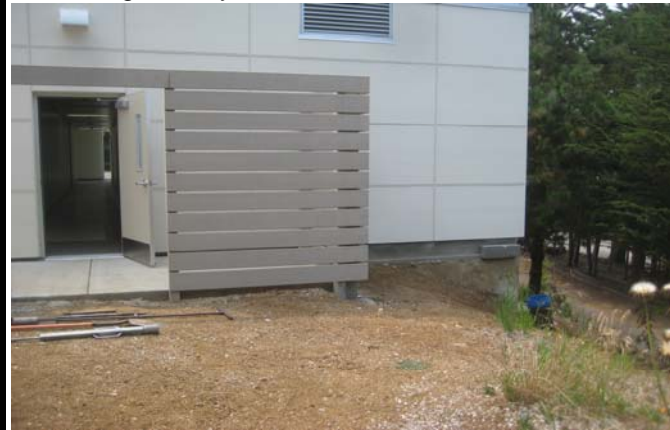
21- Loose soil adjacent to the building
