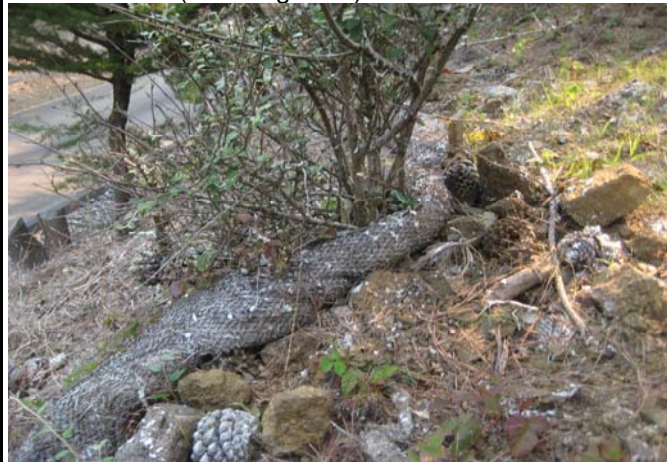
11- Soil Erosion - North Side - Caving
