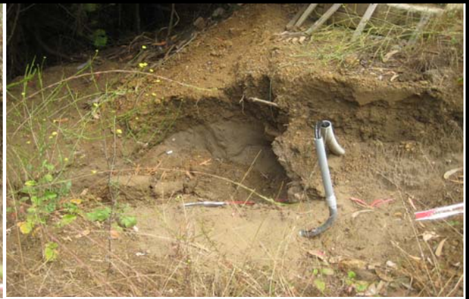
20- Utility trench erosion
