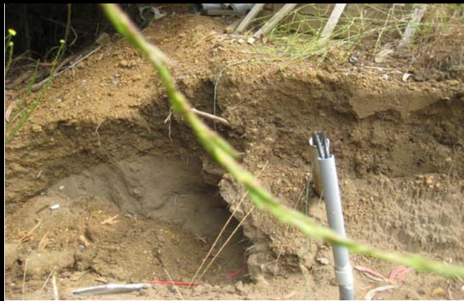
19- Caving of utility trenches - Erosion
