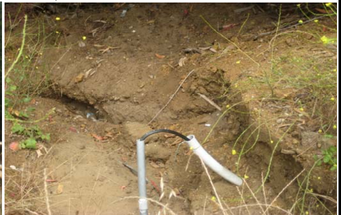
22- Erosion of utility trenches
