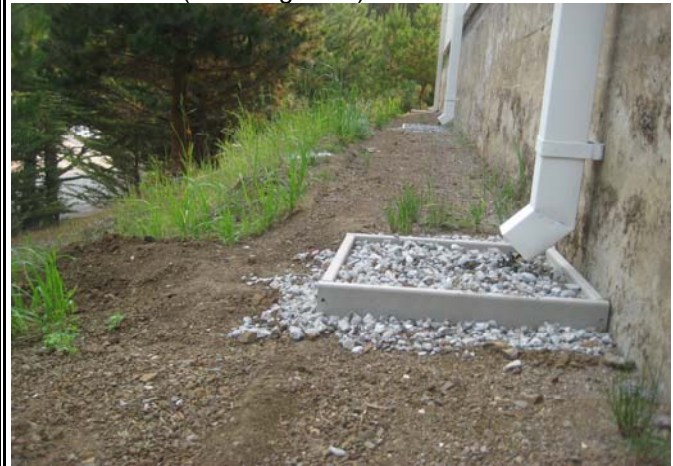
5- Soil Erosion - North Side - Caving
