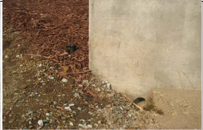
2- Drain from equipment washing area
