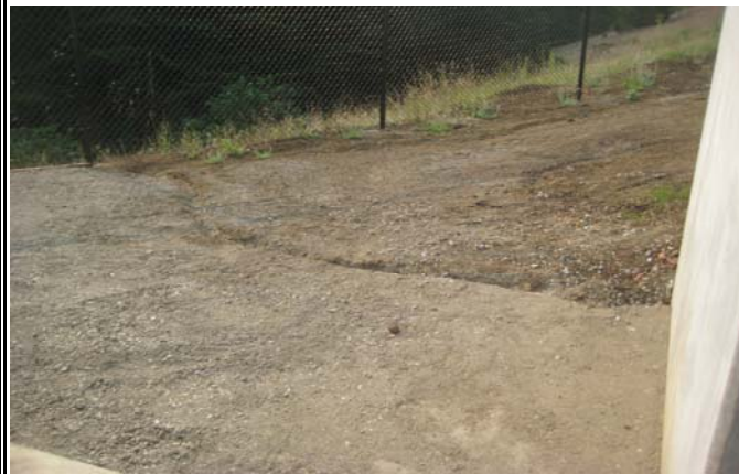
15- Loose and uncompacted soil on the south slope
