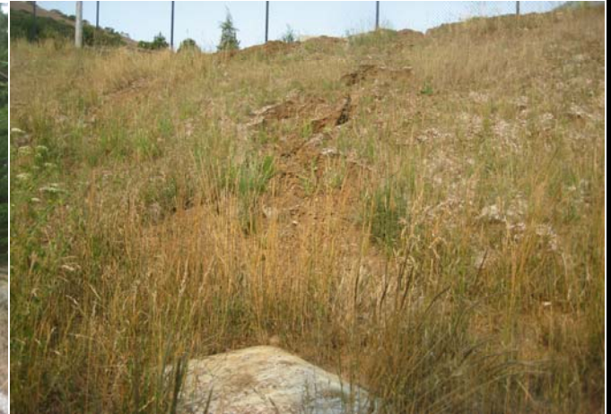
24- Slope erosion south - east of the property
