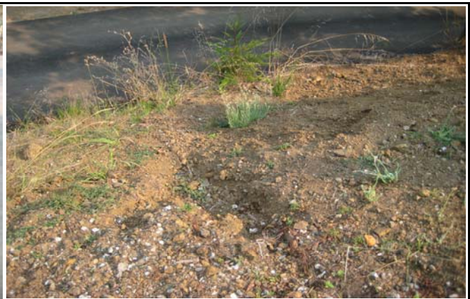
14- Soil erosion on the north slope
