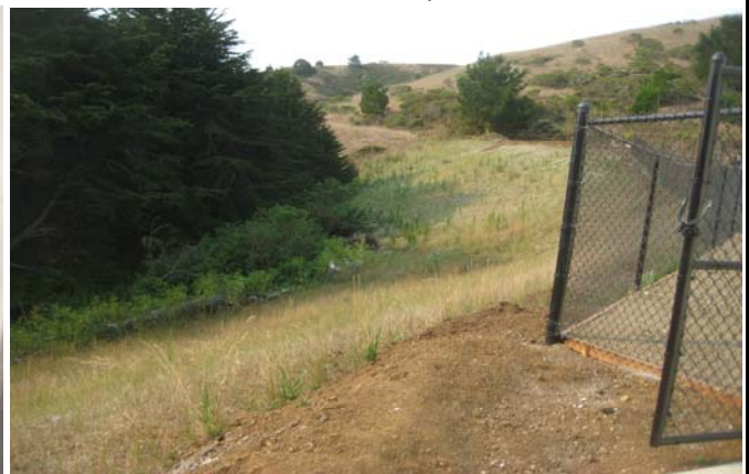
16- Soil erosion-drain outlet - east slope
