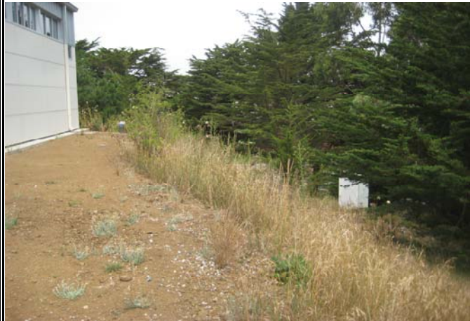
17- Soil erosion - east side
