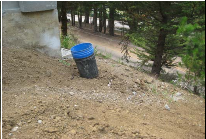
18- loose, uncompacted soil on the north slope
