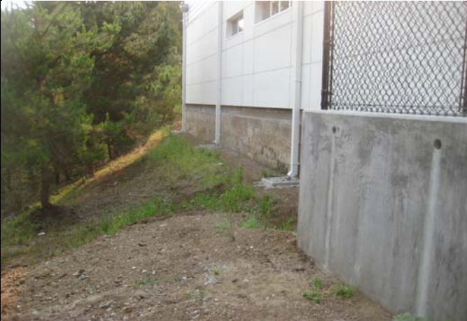
9- Drain outlet (Washing Area) - Soil Erosion
