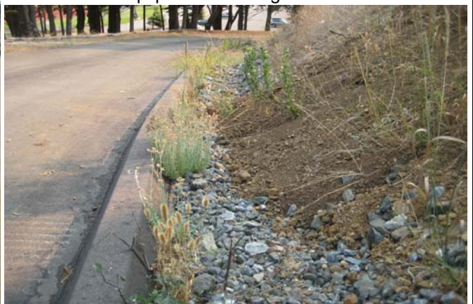
4- Soil Erosion - North Side
