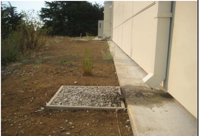
10- Soil Erosion - North Side
