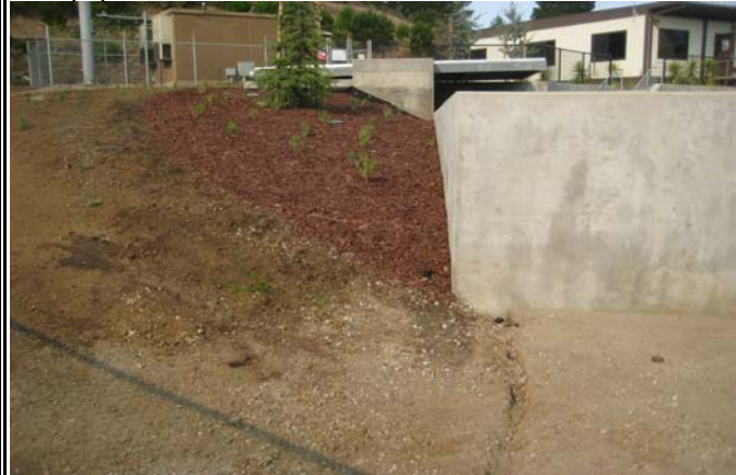
3- Drain outlet (Washing Area) - Soil Erosion
