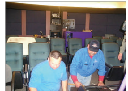
Moe Garza and Tim Granillo's precise installation of the projector stand enabled work to continue on the new projector.
