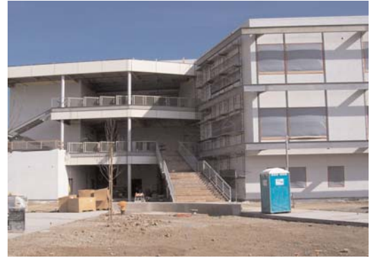
New Library and Student Resource Center (Building 9) Under Construction at Cañada College
